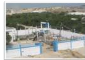
Sewage Pumping Station and wastewater networks
