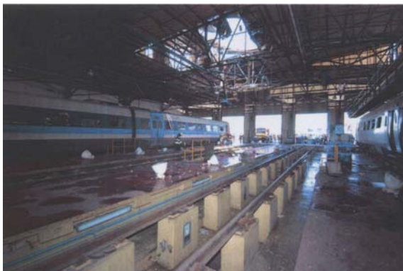
The hole in the roof where the rocket hit
