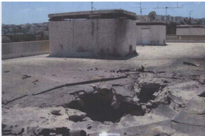
The roof of a building in Haifa – the rocket penetrated three floors.
