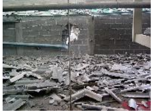
Asbestos-containing debris which fell from the roof of a factory hit by a rocket. Dozens of buildings whose roofs were made of asbestos and asbestos-containing cement were hit by Hezbollah rocket fire. The rocket fire led to the release and dispersal of carcinogenic asbestos fibers into the air.
